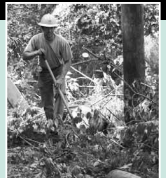
Some called it a "microburst," some just called it a bad storm. Whichever it was, the July 27 event caused significant damage and power outages for WEC members in Brookfield. Page 2.
