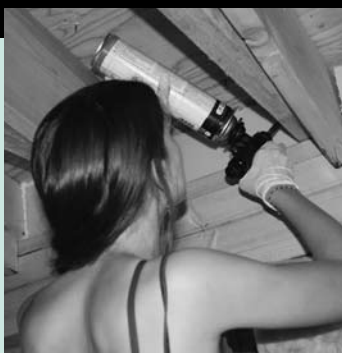
Lillian Alexander of Cabot applies pink board and caulk to tighten up an air leak at an East Montpelier home. Lillian was one of nine area students involved in July’s Summer Energy Camp. Story on page 1.
