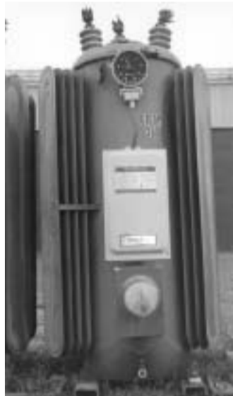
This big daddy is a voltage regulator. Positioned at a substation or out on the lines where voltage starts to weaken, voltage regulators keep the current at full strength.
