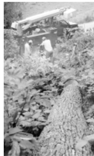
Trees down and power lines down. It happens. But it's tough for everyone when it happens to transmission lines.
