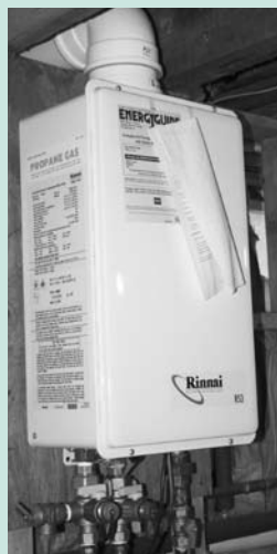
A wall-mounted, tankless, LP-fired water heater. This item, in the Mason-Sherwood home in Corinth, has cut their power bill more than in half. Their page 1 story continues inside.
