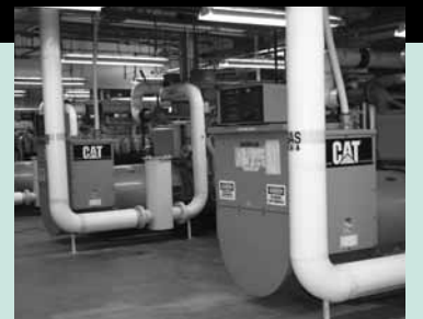
A couple Caterpillar engines at Washington Electric's generation plant in Coventry, Vermont. Tours of the plant have been popular, and now you can take one from the comfort of your easy chair. Page 2.
