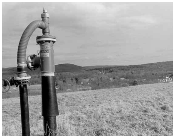
A wellhead at the New Milford, Connecticut, landfill.
