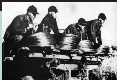
The "Four Horsemen of the Lines," a famous photo of workers spooling out power line in a mad dash to complete construction one day before the Brown-Atchison Electric Cooperative of Horton, Kansas was energized on March 31, 1938. Photo courtesy of the NRECA.
