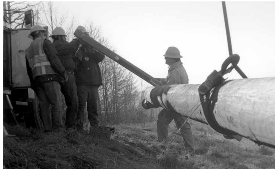
The Coventry project necessitates construction of 7.4 miles of transmission line to a VELCO substation. Here, workers from Eastern Utilities Inc. prepare to set poles.
